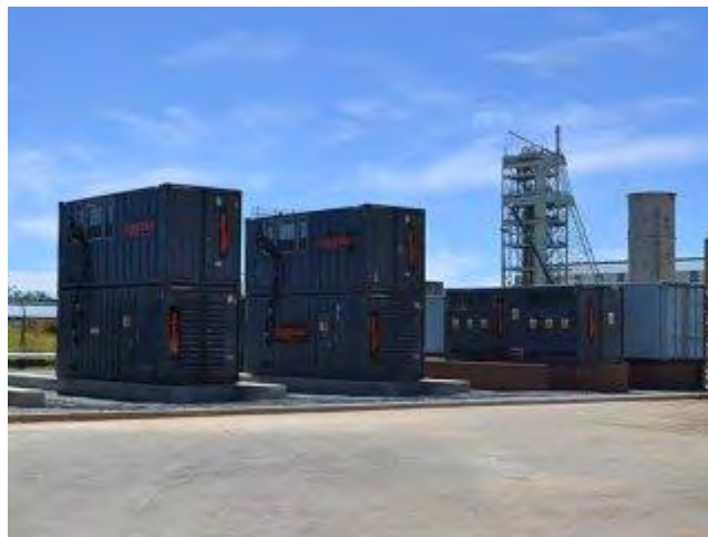
Figure 48: Generator set at Mine C gold mine (Creamer, 2013)
