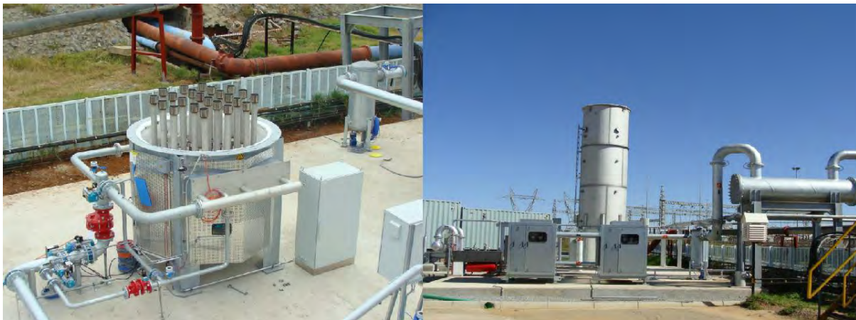
Figure 47: Methane burner at Mine C
