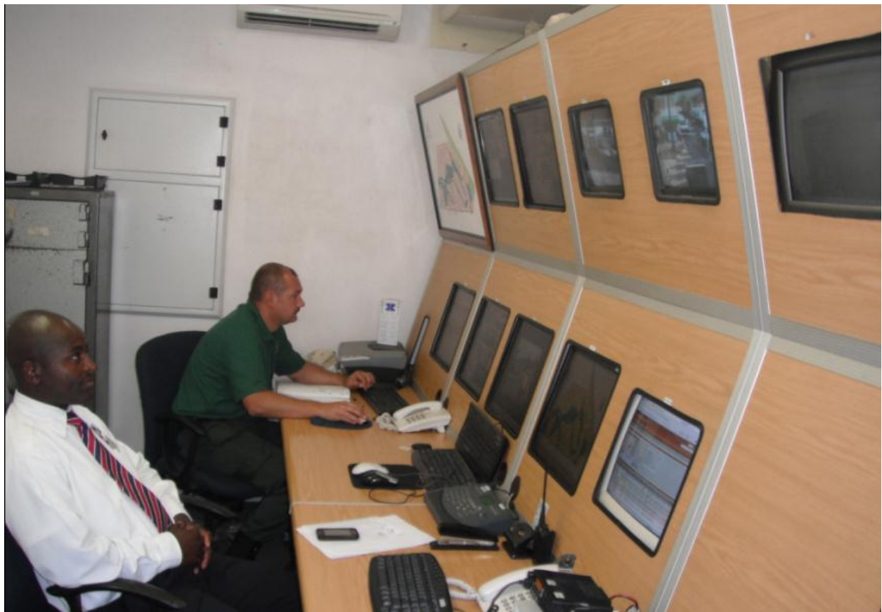
Figure 11: Silver Lakes Golf Estate control room
