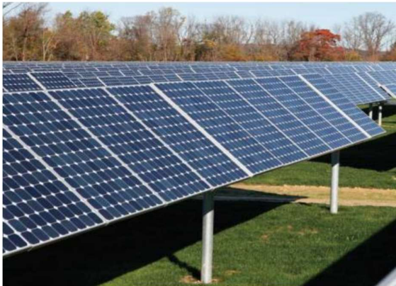
Figure 3.1: Example of a horizontal single-axis tracking
