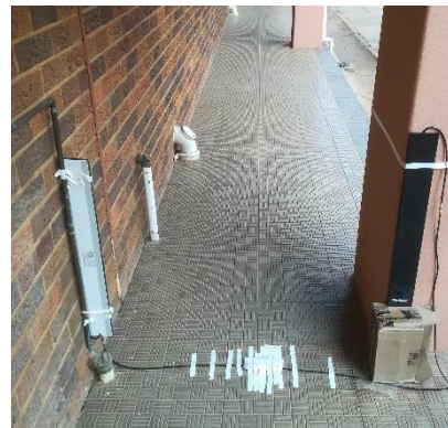
Figure 3-9: Antenna installation on both sides of a passageway
