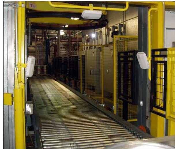
Figure 2-23: Typical 3 antenna setup inside a bay door, reproduced from [74]
