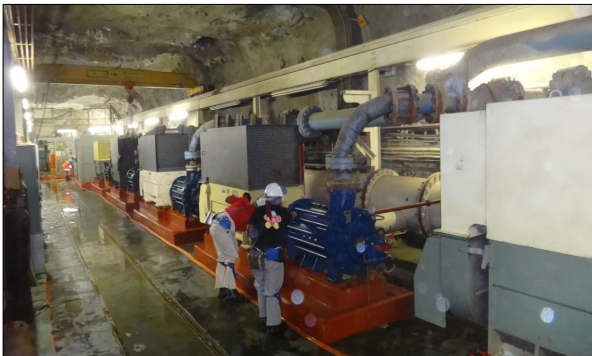
Figure 25: Mine dewatering pump station 12
