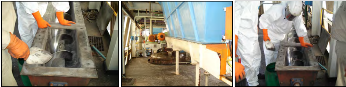
Figure C5. VRP . Cleaning dust extraction fan filters (3.242 g/m 3 )
