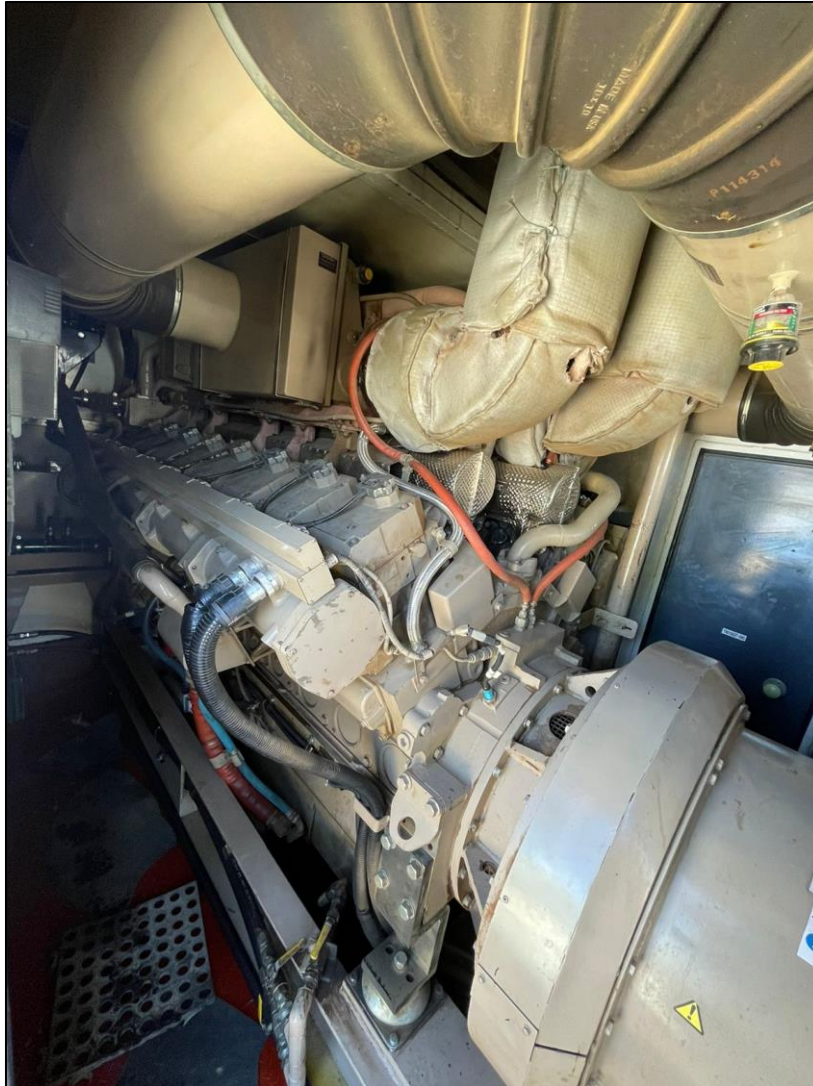
Figure 24: Methane-fuelled SI engine at a deep-level mine 2
