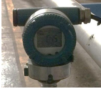
Figure 73: Pressure indicator at UF inlet
