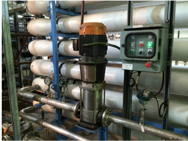
Figure 76: RO1 inter-stage booster pump
