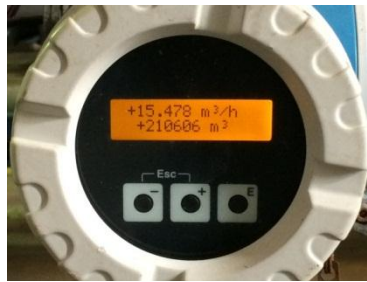
Figure 80: Flow meter of RO1 brine
