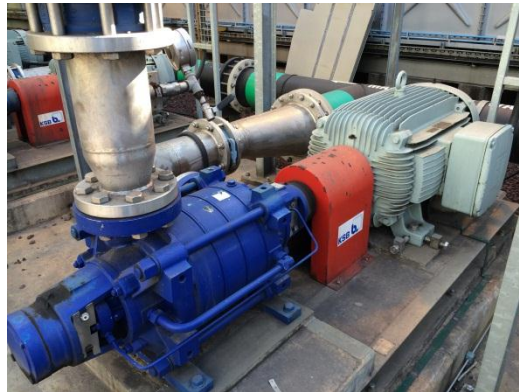
Figure 75: RO1 high pressure feed pump
