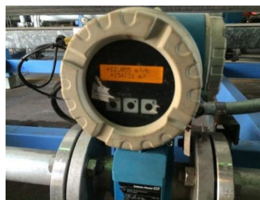
Figure 84: RO2 brine flow meter
