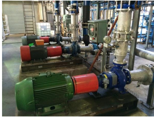
Figure 85: CEDI booster pumps
