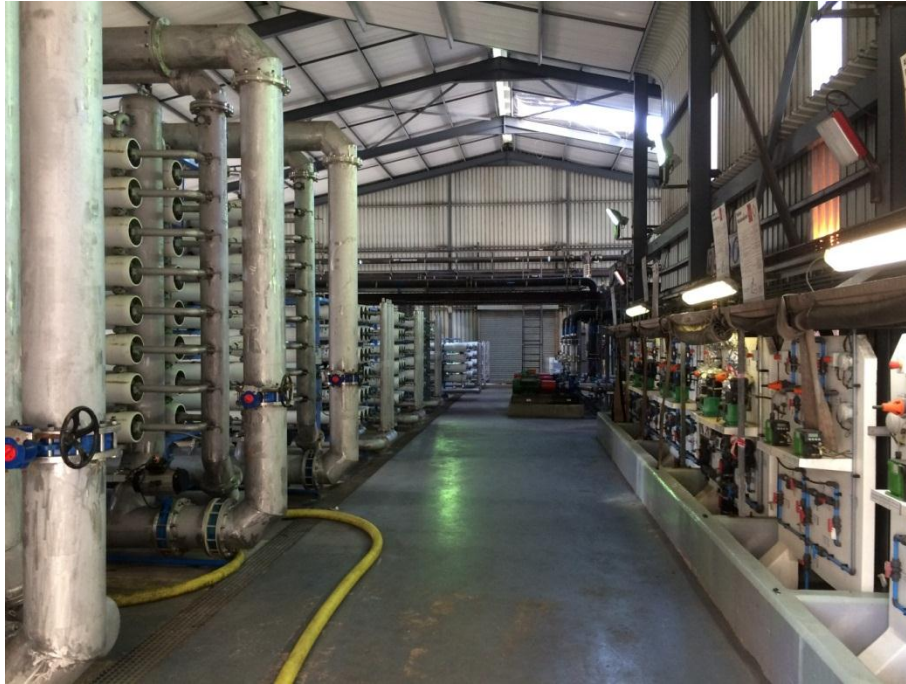
Figure 71: Desalination plant with UF skids, first and second RO stages and chemical dosing stations
