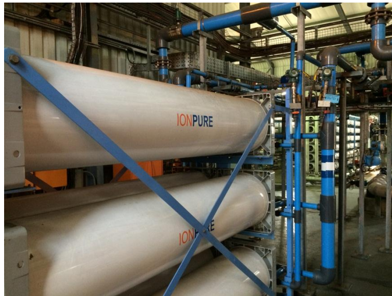
Figure 29: CEDI modules under investigation
