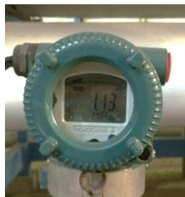
Figure 78: Pressure indicator after the RO1 booster pump
