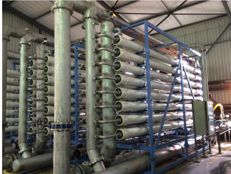
Figure 24: UF skids installed on the plant under investigation
