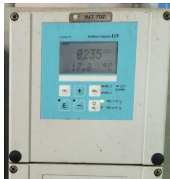
Figure 74: Turbidity analyser after UF membranes
