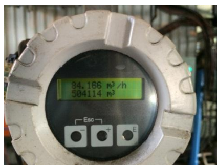
Figure 87: Flow meter on CEDI permeate
