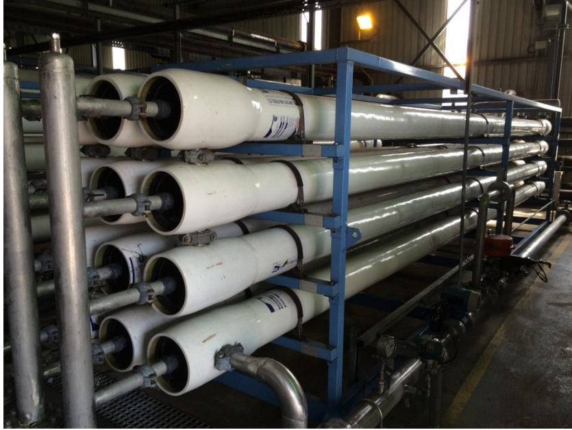
Figure 28: Second stage RO on the plant under investigation
