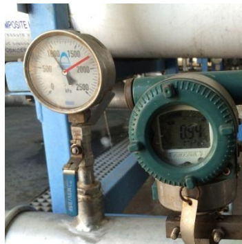
Figure 83: RO2 brine pressure indicator
