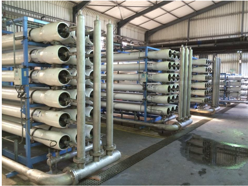
Figure 27: First stage reverse osmosis skids 1, 2 and 3 in the investigated plant
