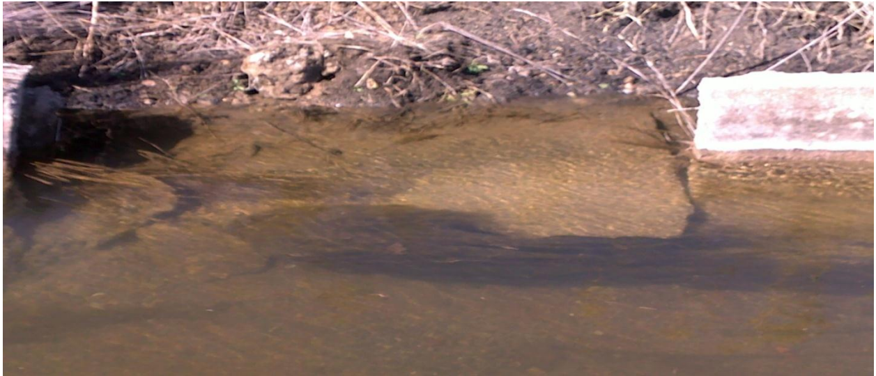
Photograph 4: Mooibank canal structural failure (fallen wall), Haaskraal
