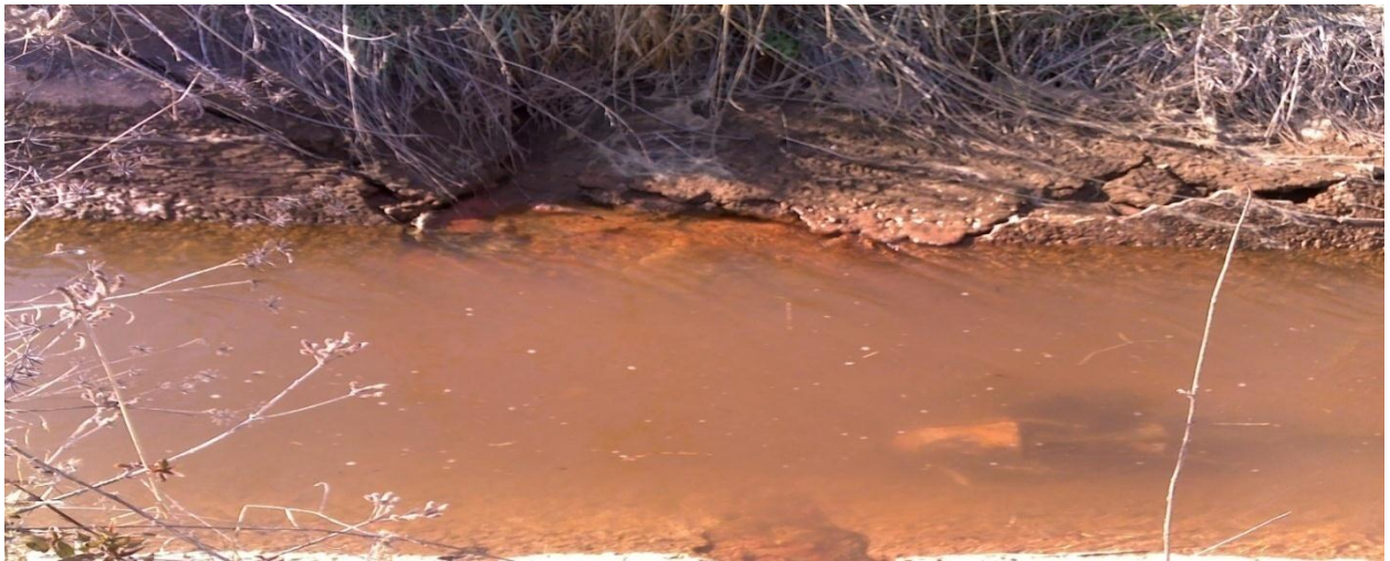
Photograph 5: Mooibank canal (structural failure) with flowing dirty water Haaskraal (Photographer:
