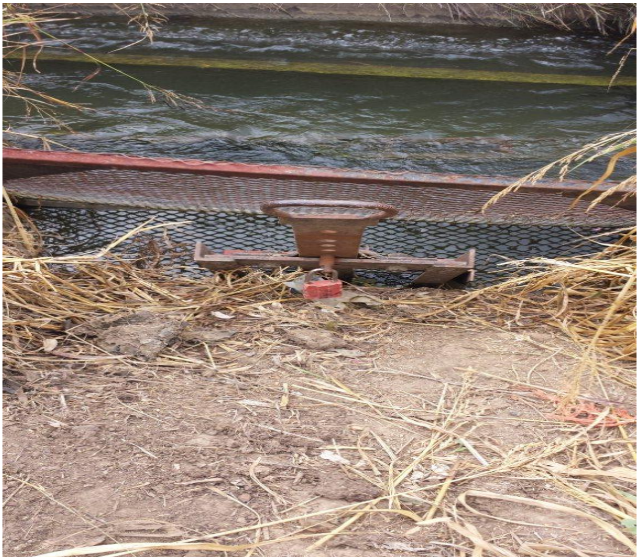
Photograph 8: Mooibank illegal abstractions (Sluice with a broken padlock)
