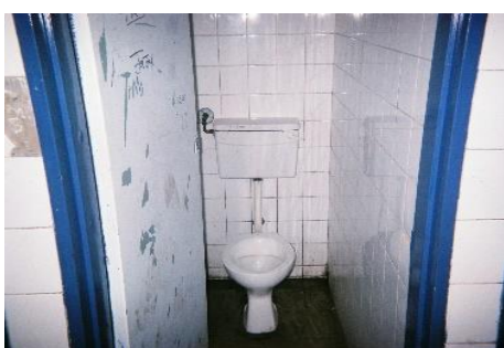
Figure 6. 28: Dirty toilet falling ceiling board
