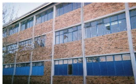
Figure 6. 27: Broken windows in classrooms
