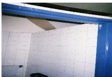
Figure 6. 29: Toilet with broken ceiling
