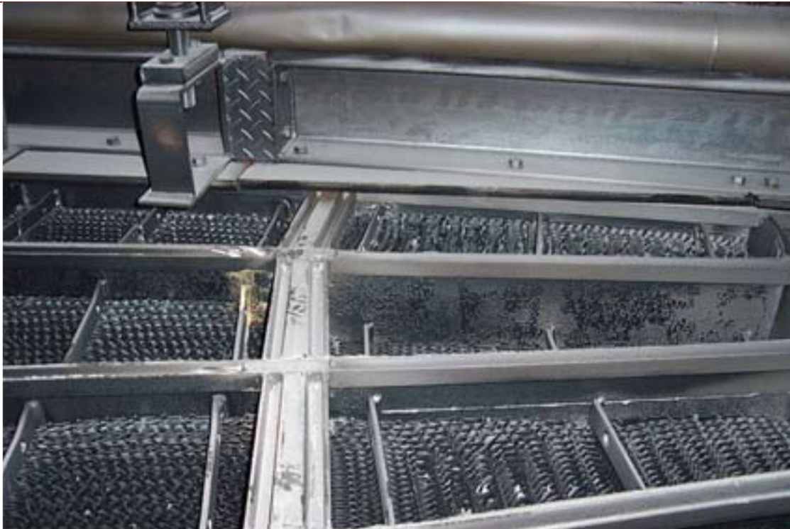
Figure 8 : Cast iron wear shoes installed (Howden,2014)
