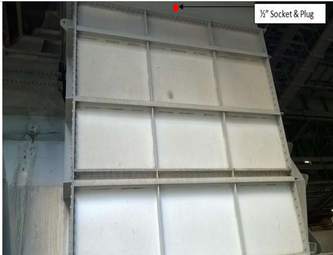
Figure 21 : FD fan suction test point
