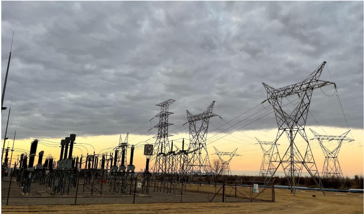
Figure 10: Mine substation point of supply 7
