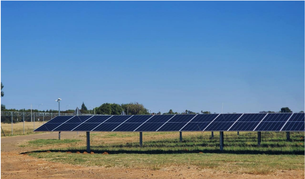
Figure 23: Solar PV arrays at a mine solar farm 11
