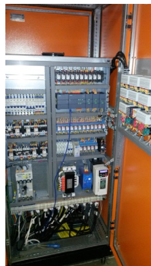
Figure 4-2: (a) Exterior of the universal test panel for use of testing pilot plants with a maximum output amperage of 1150 Amperes, and (b) control circuitry within the universal test panel
