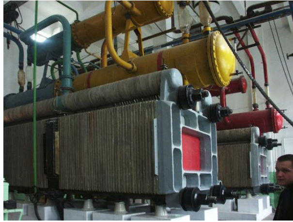
Figure 2-18: Typical gas/liquid separator scale located above a 500 Nm 3 /hr alkaline water electrolysis plant [16]
