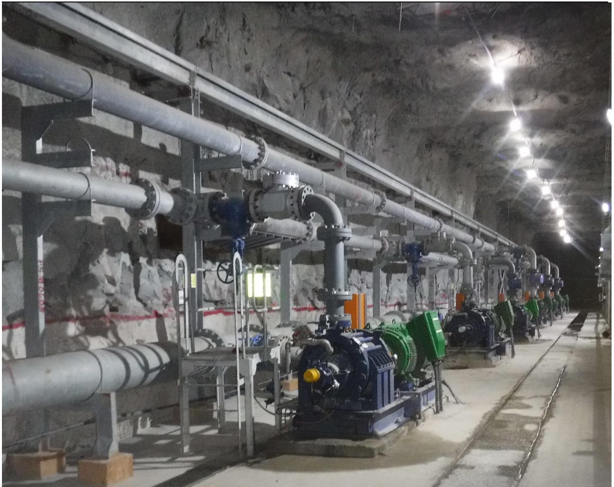
Underground pump chamber 3
