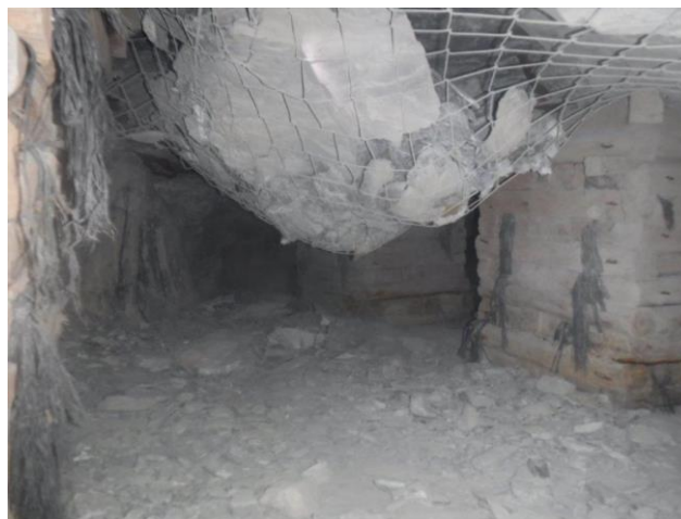
Figure 3: Chain link wire mesh deflection after fall of ground
