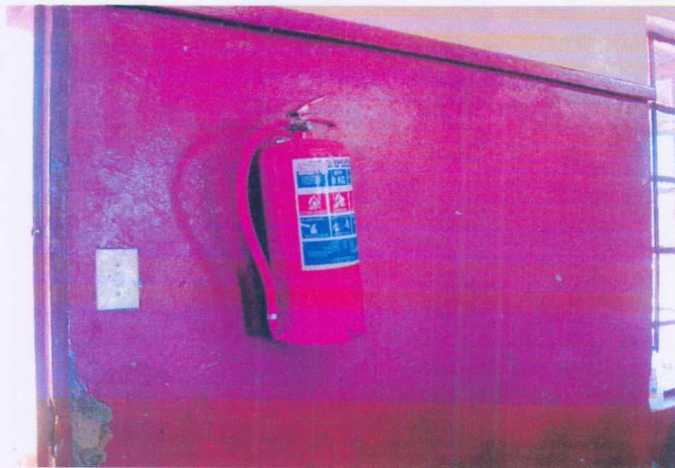
Figure 4.18: A fire extinguisher at a school
