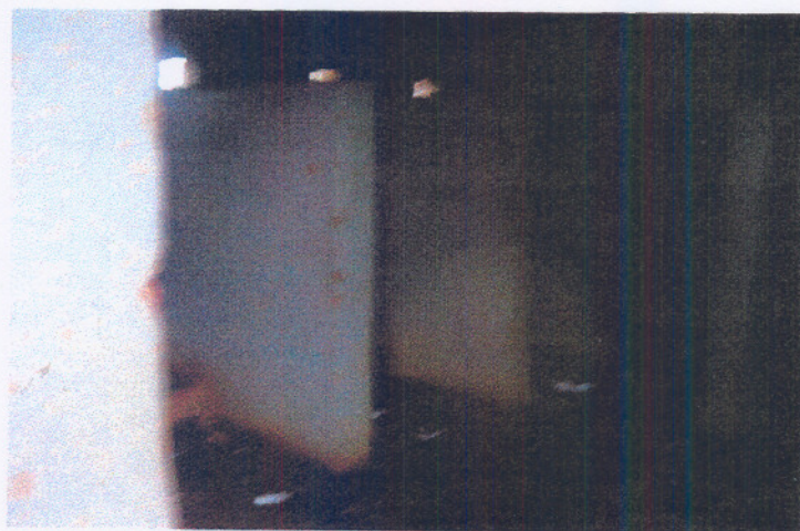
Figure 4.3: Unhealthy and unsafe school toilets
