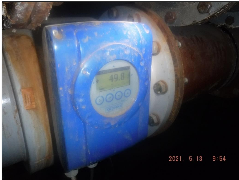
Figure 41: Water flow meter at Shaft A
