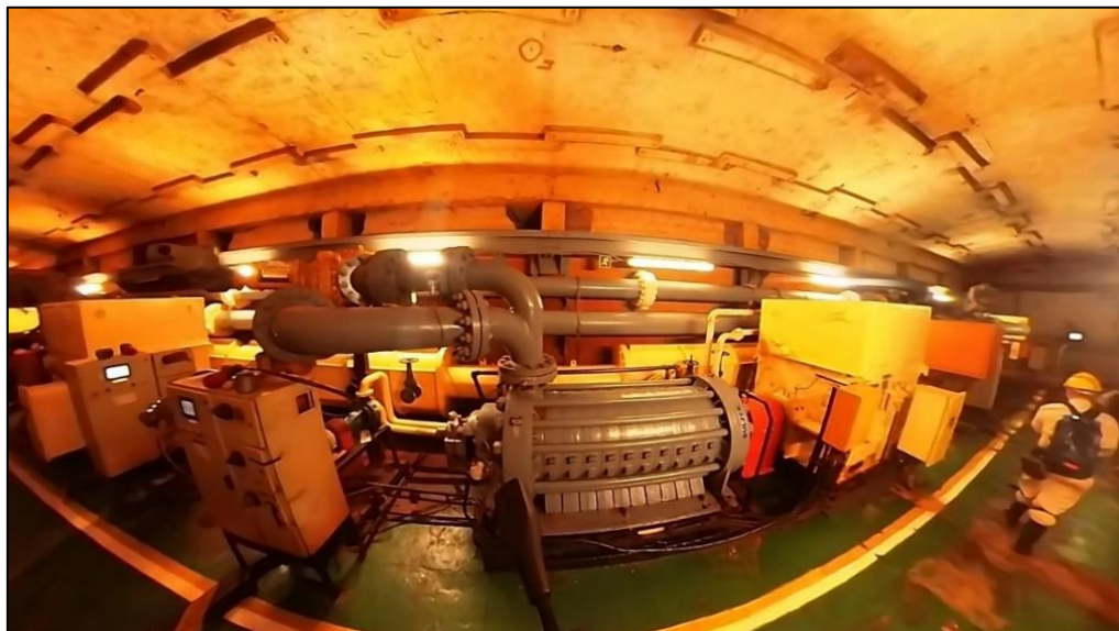
Figure 37: Underground dewatering pump
