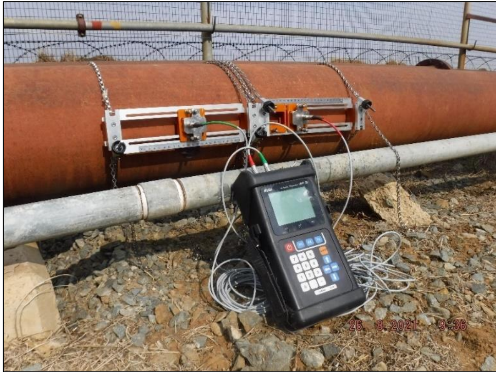
Figure 14: Clamp-on ultrasonic flow sensor [118]
