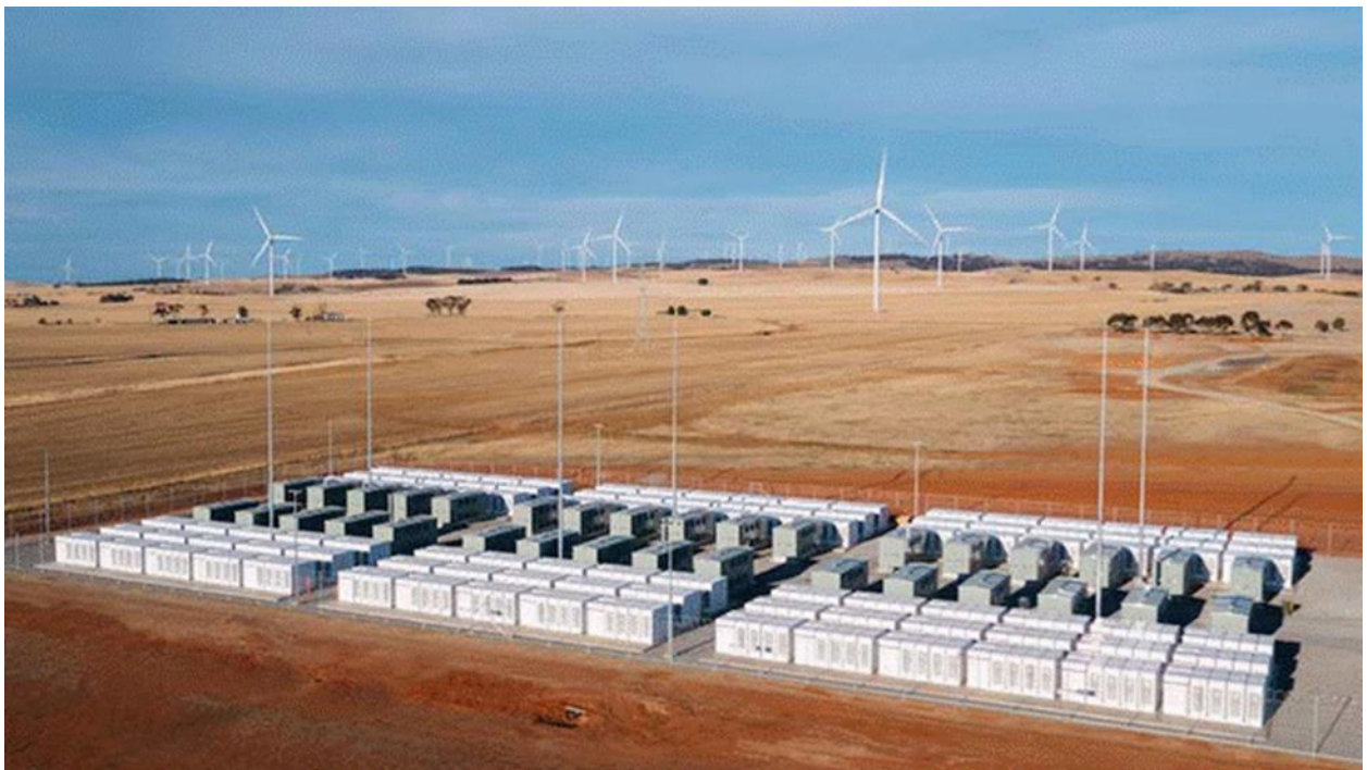
Figure 2-21: Hornsdale wind is South Australia,
