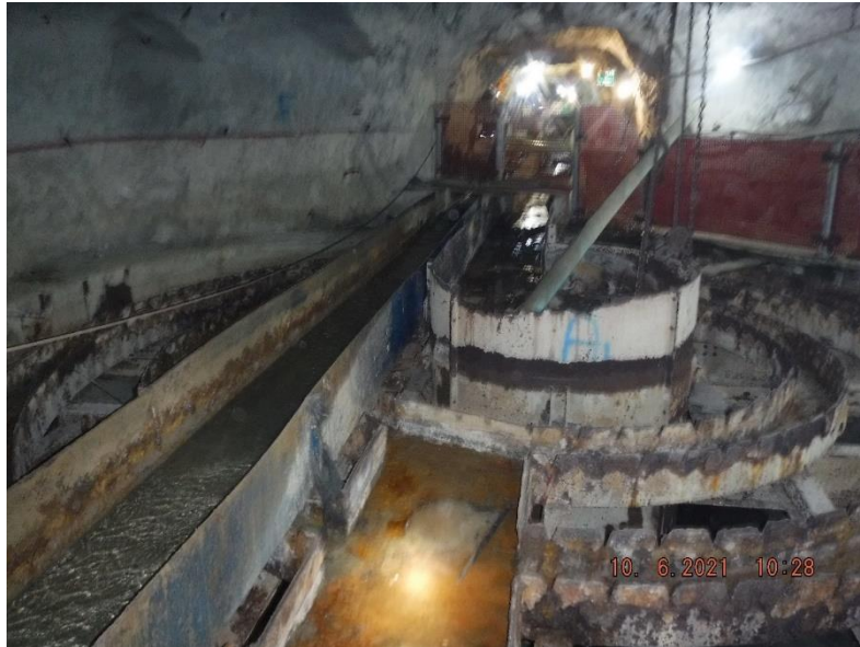
Figure 72: Empty settler with a drain manifold constructed to allow water to flow past
