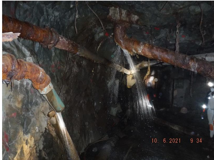
Figure 66: Pipe configuration with leakages and unfinished sections
