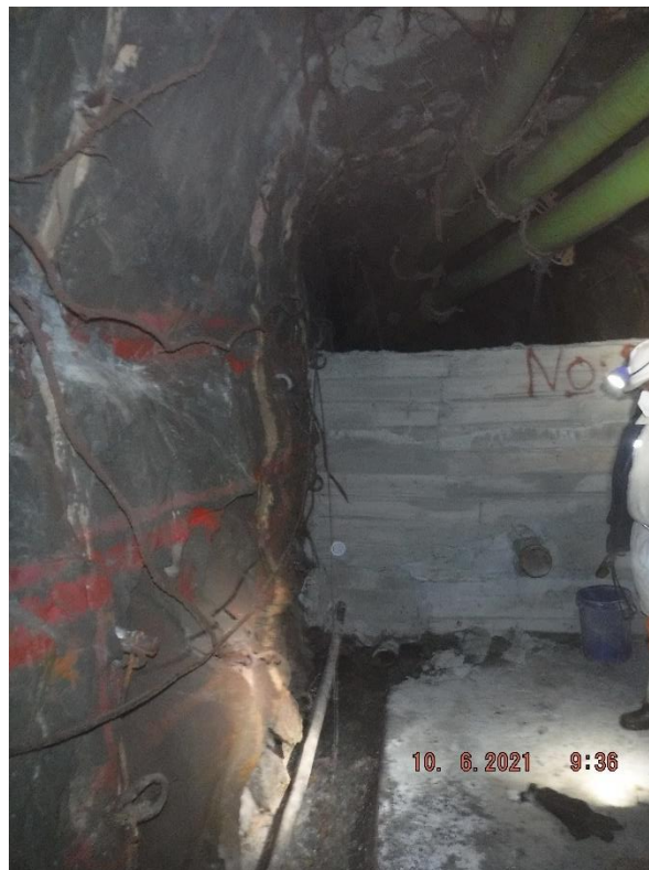
Figure 71: Emergency dam created by closing off a haulage section
