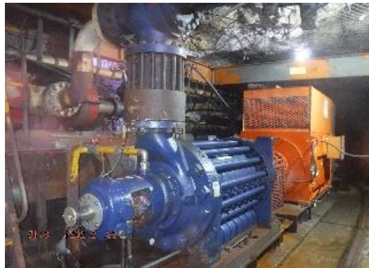
Figure 60: An 11 MW mine dewatering pump
