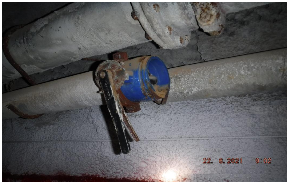
Figure 65: Unfinished pipe with a closed butterfly valve
