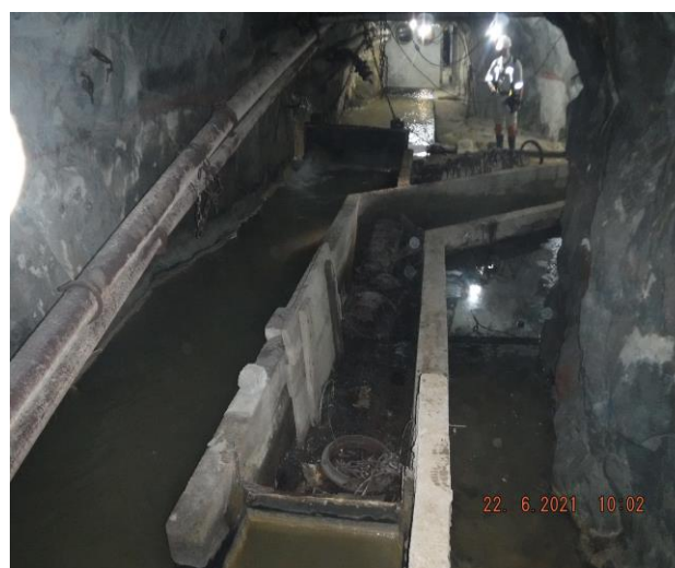
Figure 63: Settler area inlet drains
