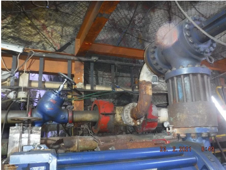
Figure 68: Dewatering pump outlet pipe manifold with valves
