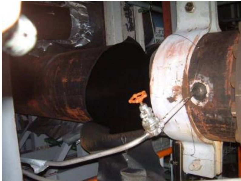
Figure 1 – Pipe rupture on a nuclear plant (Corrosion Doctors, 2011)
