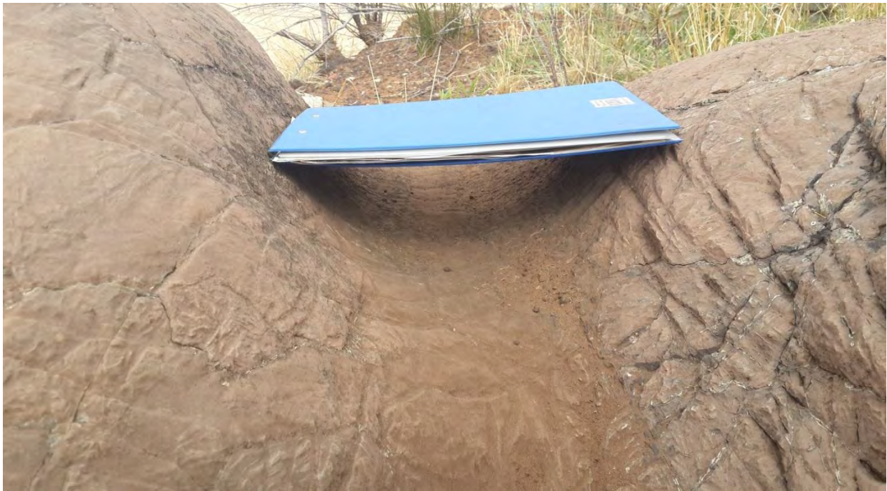
Figure 82: Photograph showing a shallow hole present on the surface of the Oaktree Formation dolomites in the study area. Photograph taken by Daniell (2014).
