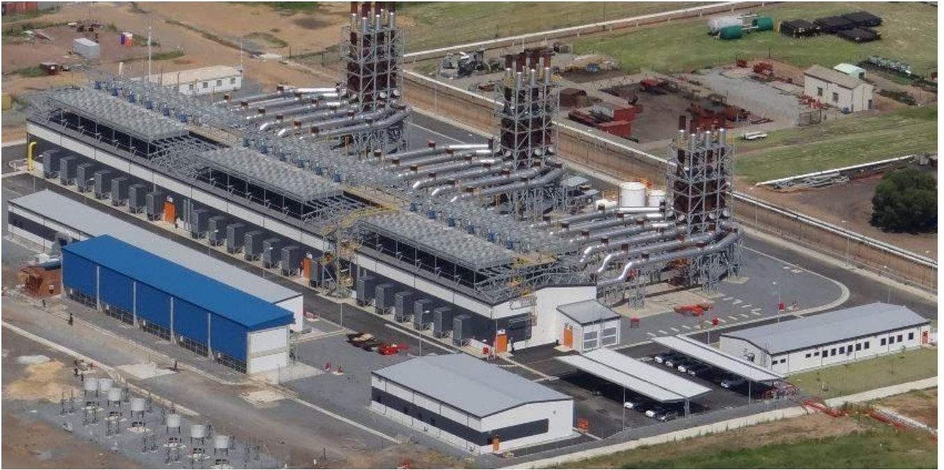
Figure 1.1: Sasol Gas Energy Power Plant, Sasolburg
