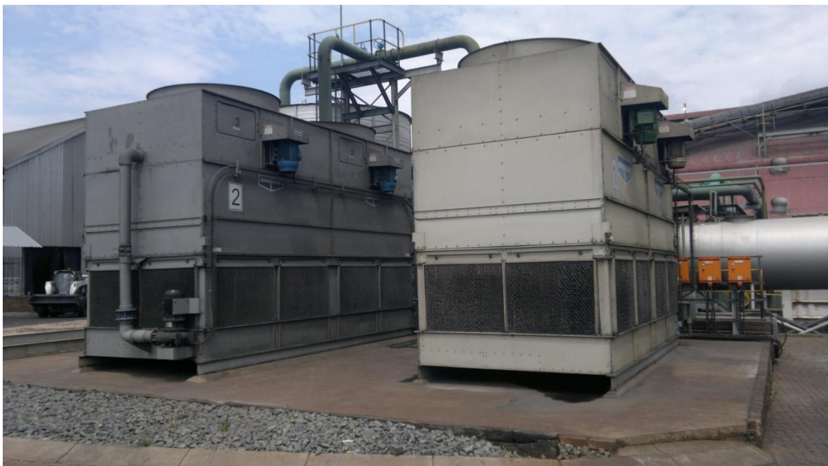
Figure 14: Closed circuit cooling towers
