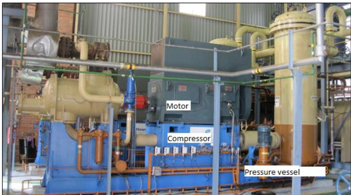
Figure 13: Practical example of a chiller machine
