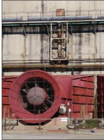
Figure 15: Practical example of a bulk air cooler
