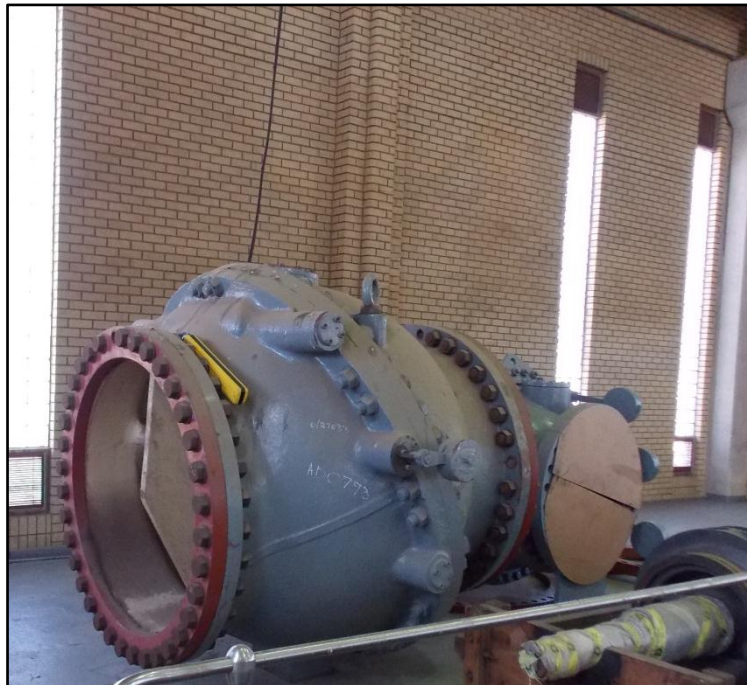
Figure 25: Typical valve out of commissioning
