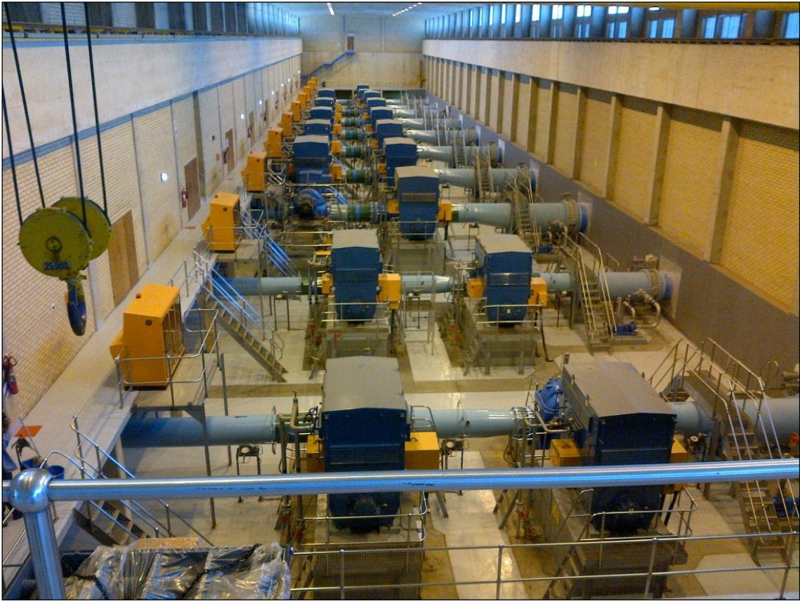
Figure 18: WTW-A Engine Room 4
