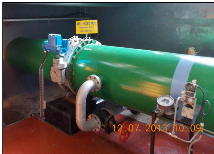
Figure 21: Typical incoming pipeline at an engine room at a WDU
