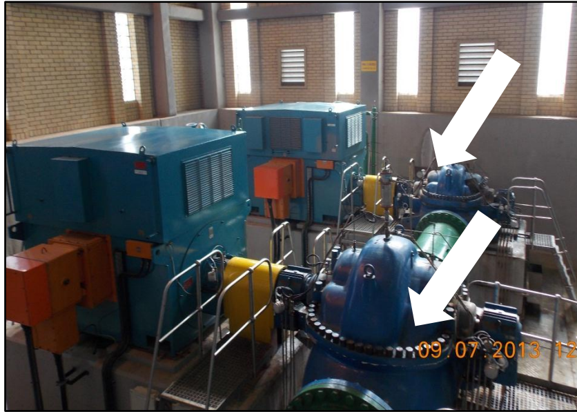
Figure 20: Typical two-stage pump set in an engine room of a WDU
