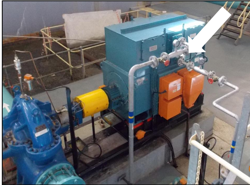
Figure 23: Pump motor connected to a pump in an engine room
