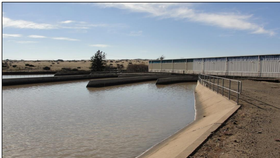
Figure 36: Inlet canal to pump station
