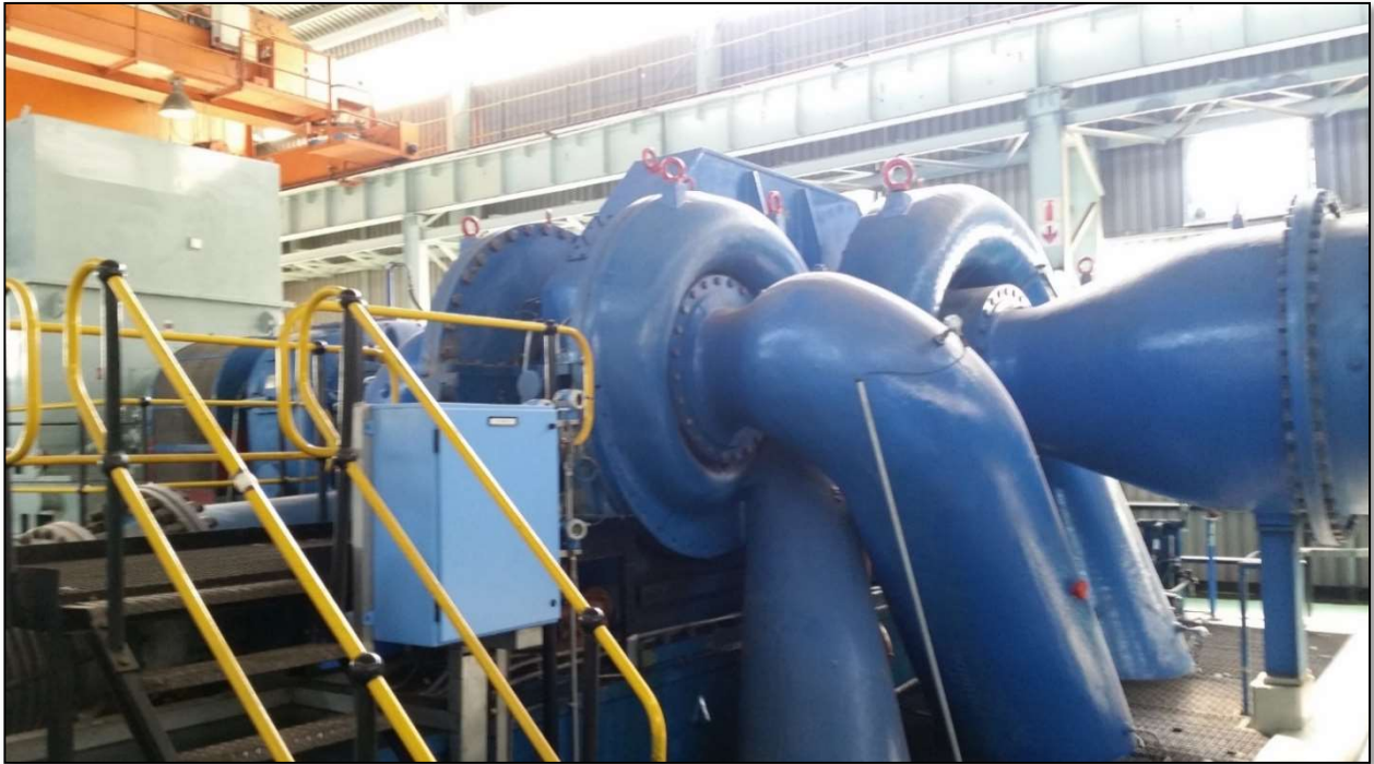
Figure 2-15: Multi-stage compressor with an installed capacity of 15 MW
