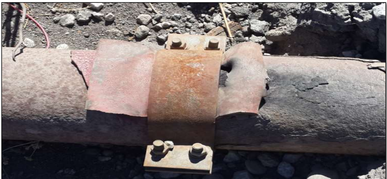
Figure 2-28: Punch leak in compressed air pipe on surface
