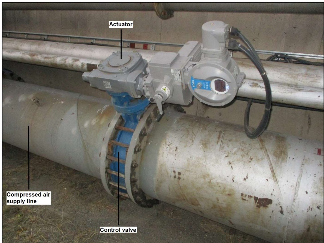
Figure 2-26: Automatically actuated valve installed on a compressed air line
