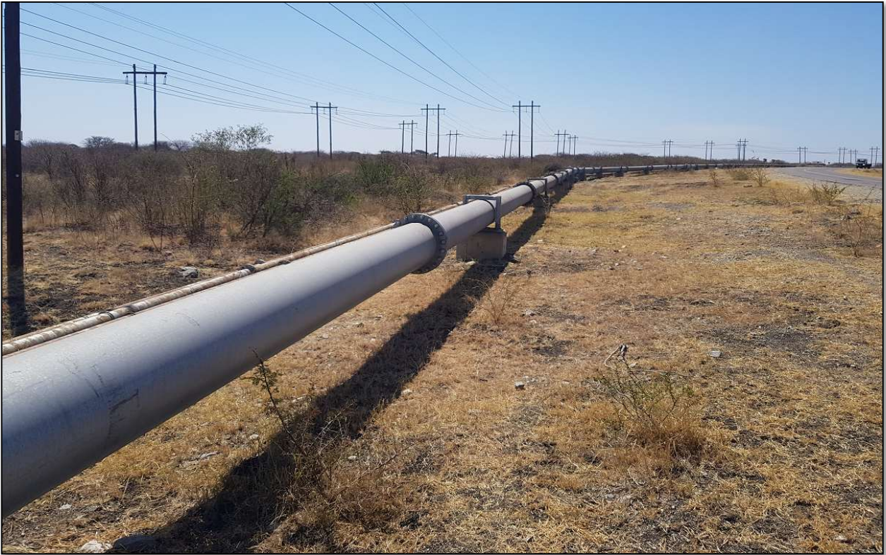
Figure 2-19: Compressed air pipe forming part of a compressed air network
