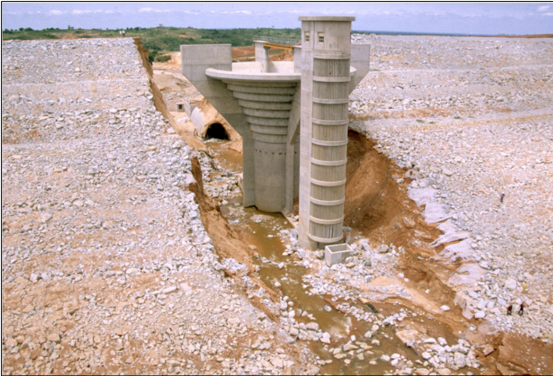
Figure 3-5: The Zoeknag Dam shortly after it failed in 1993 179
