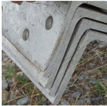
Figure 59 : Delamination of ends of members after galvanising
