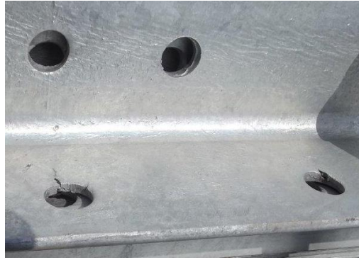
Figure 58 : Cracking and tearing of punched holes
