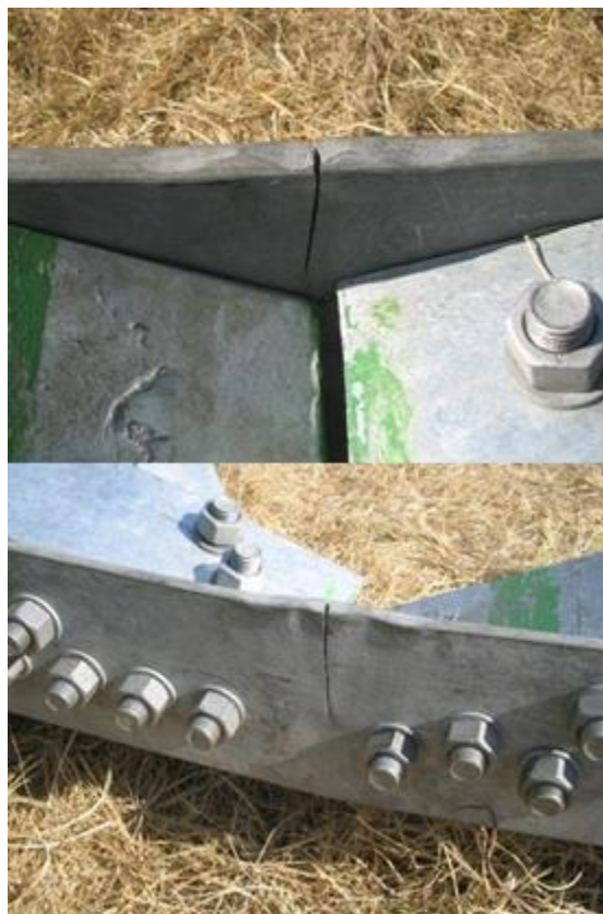
Figure 57 : Crack in bended member of K-frame
