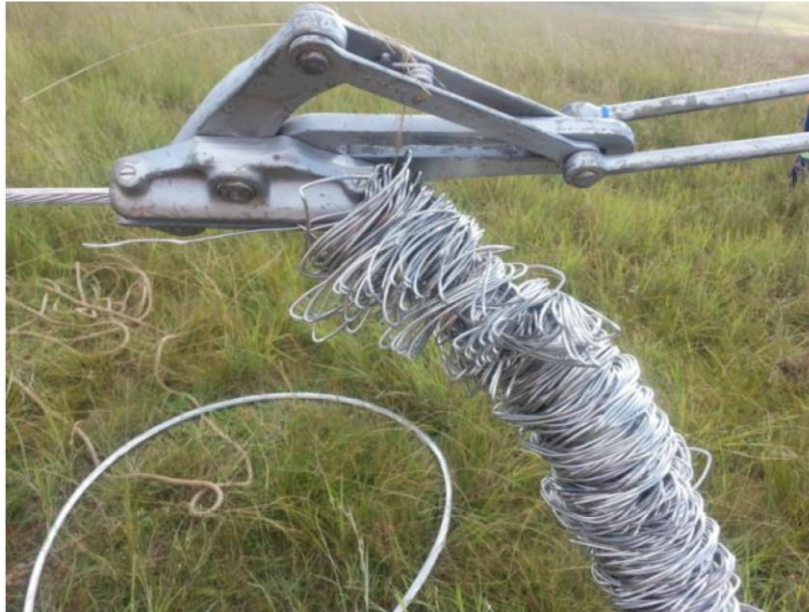
Figure 69: Slipping of a come-along clamp damaging the conductor strands
