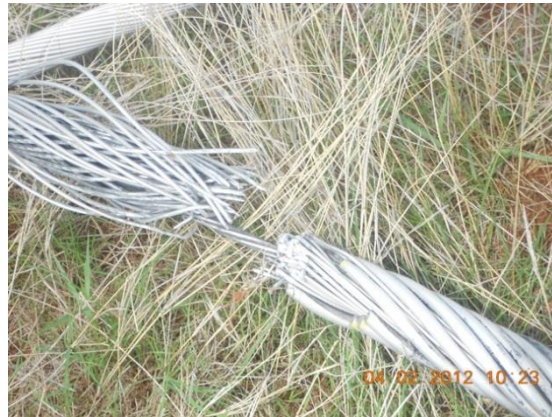
Figure 10: Fatigue damage to aluminium conductor strands
