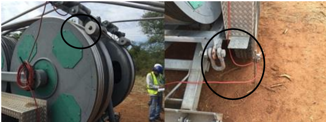
Figure 20: Running earths applied on tensioner
