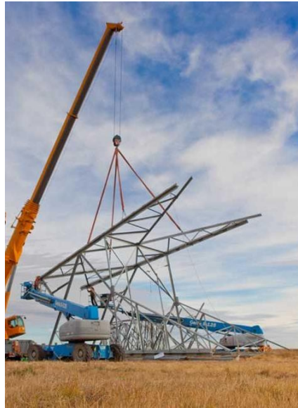
Figure 52: Foreign practice of assembling the legs of a structure as one piece before erection
