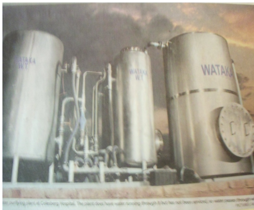
Illustration 12: This illustrates the deteriorating water infrastructure that has not been serviced for many years. The infrastructure is failing to distribute water. Source: Mercury
