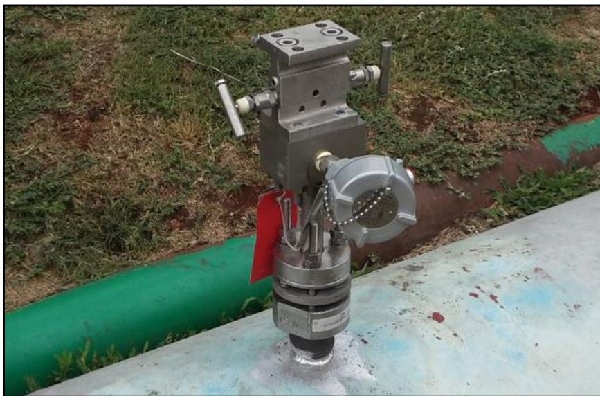
Figure 28: Actual installed Verabar® flow meter
