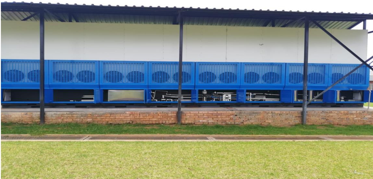
Figure 3.2: Site study AWGs front view (as per the GPS location).
