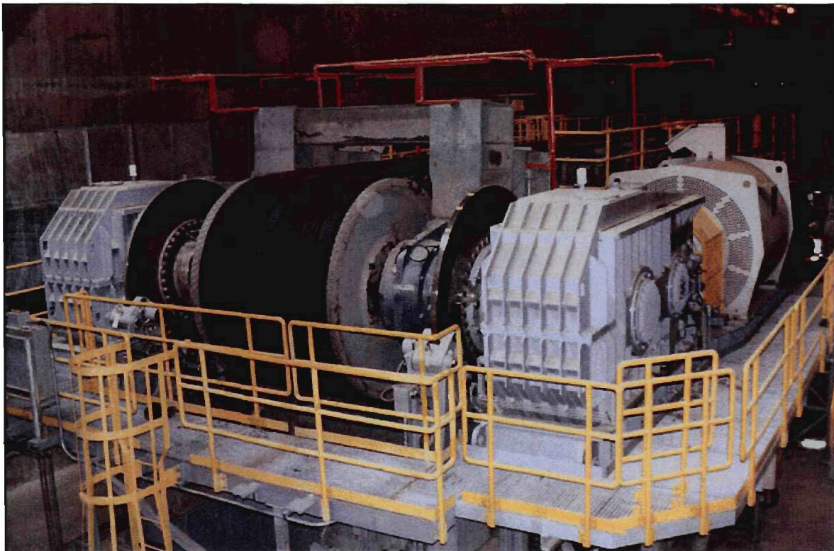
Figure 15 – Drive end for the Minera Los Pelambres downhill conveyor [42]
