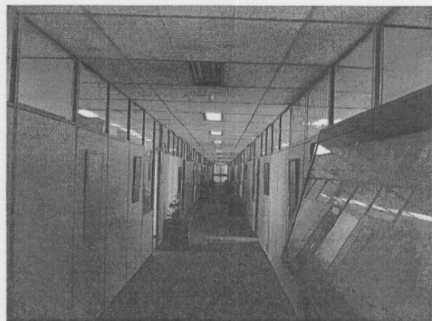
Figure 3: Typical office & hallway lighting.
