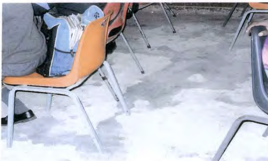
Exhibit 10 A bad floor condition
