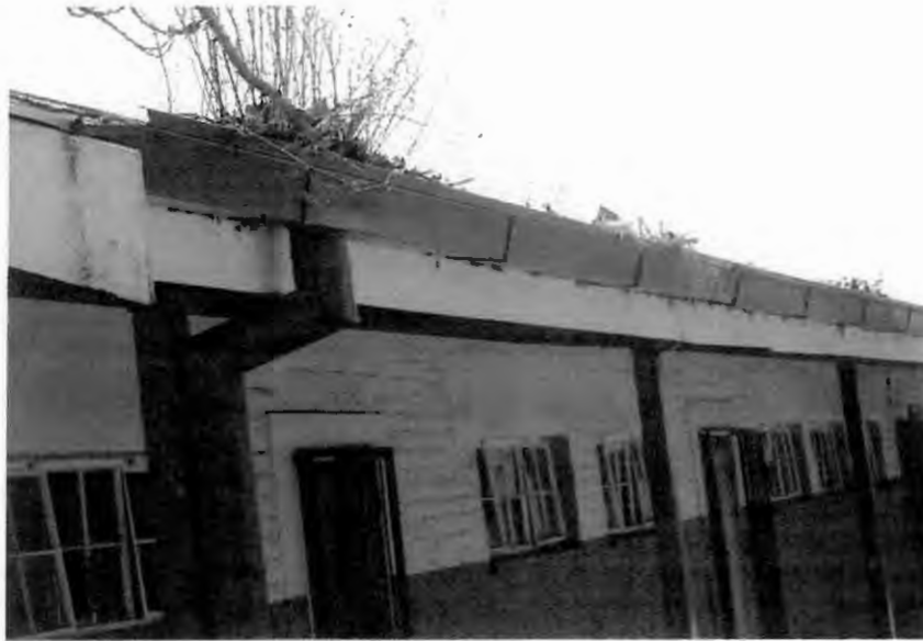
Exhibit 4 Poorly maintained gutters
