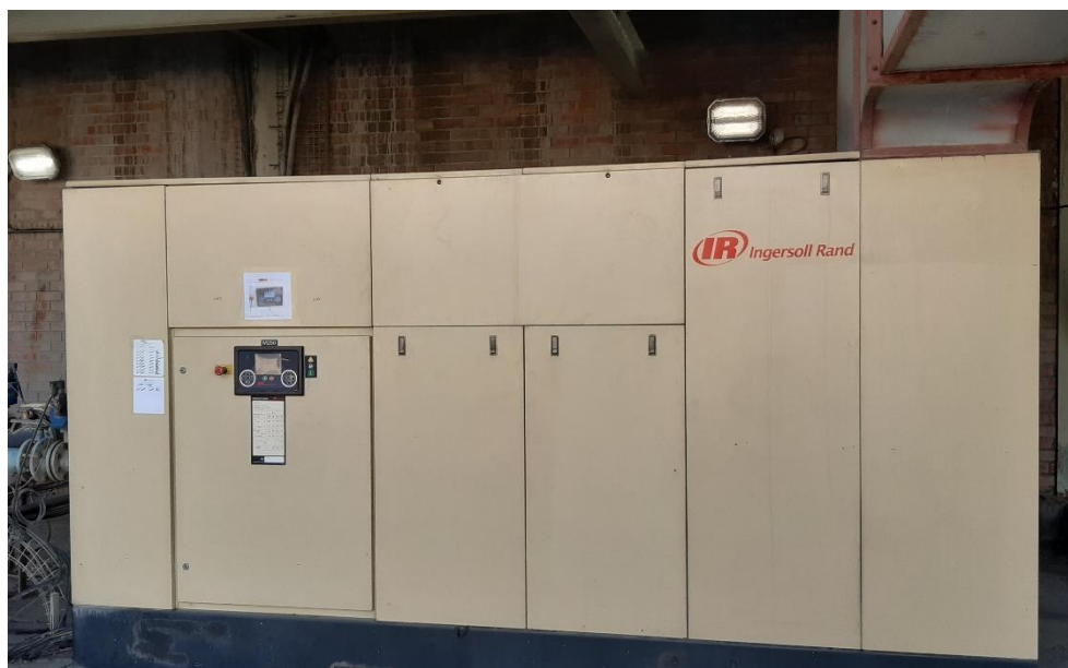
Figure 8: Platinum plant instrument air compressor
