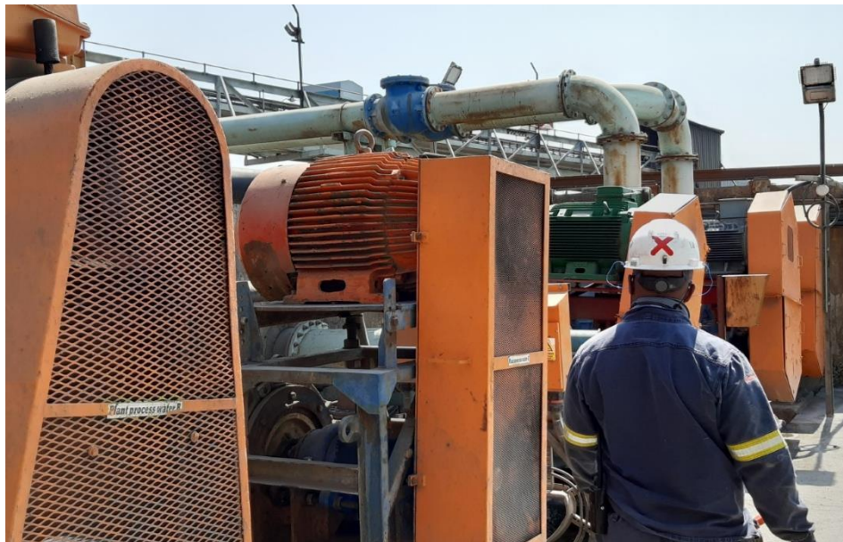
Figure 7: Platinum plant tails transfer pumps
