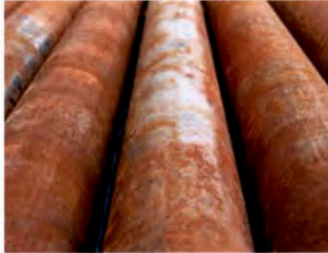
Figure 1.1: Oil pipeline corrosion [5]
