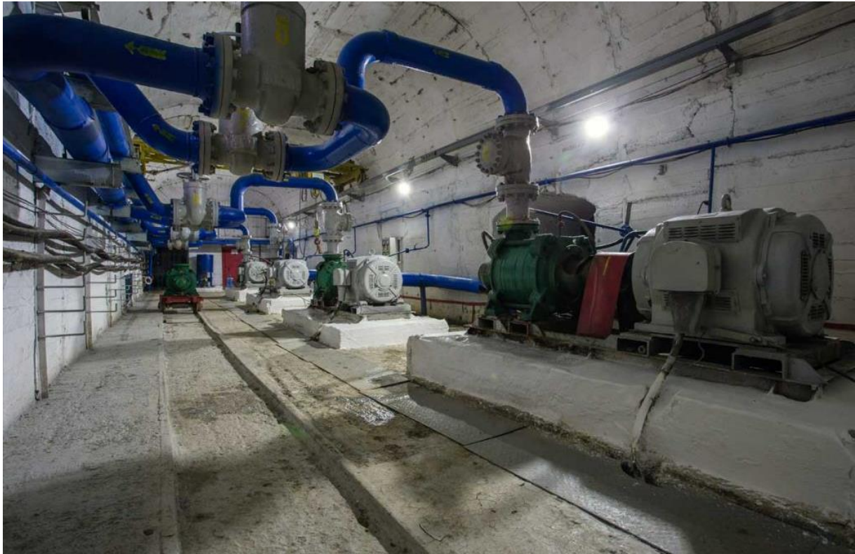
Figure 48: Underground pump chamber 4
