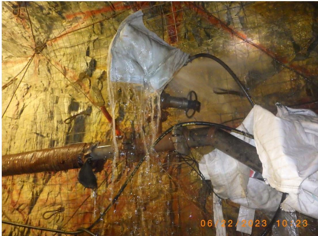
Figure 54: Leaking valve identified during implementation.
