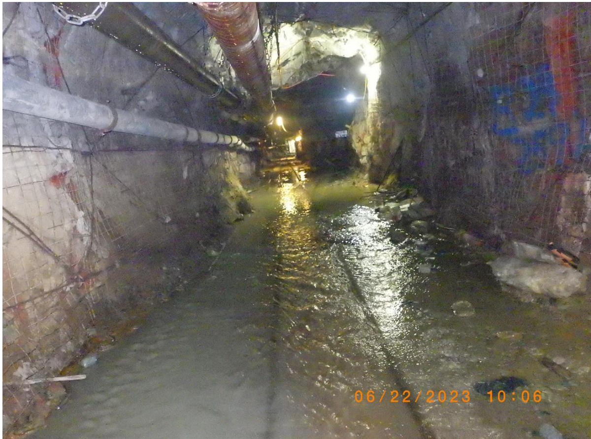
Figure 53: Flooded working area due to leaking water columns.
