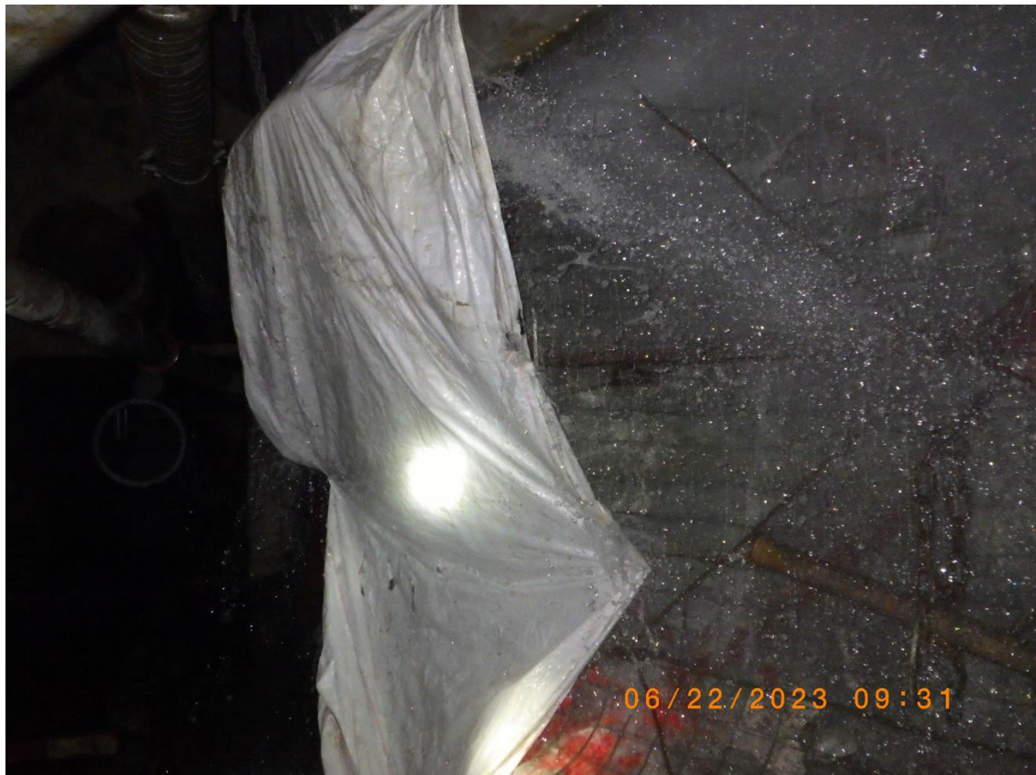
Figure 52: Burst pipe located during implementation.
