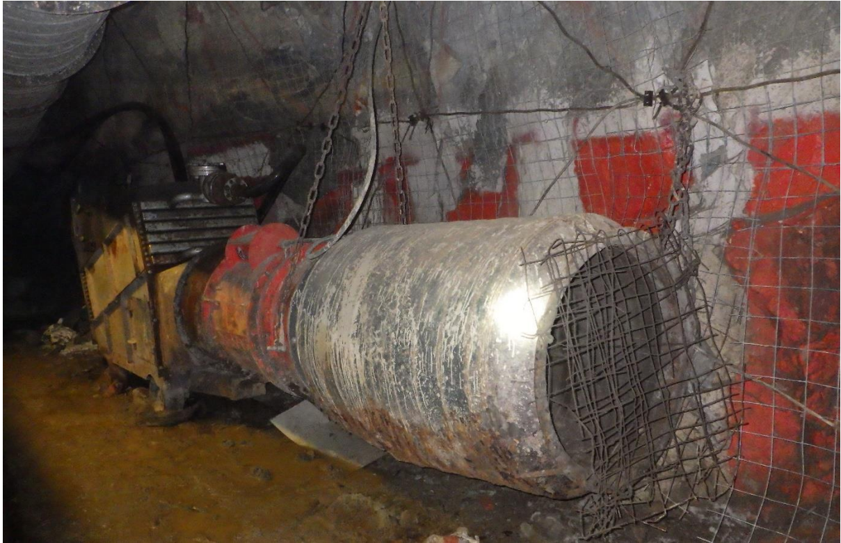
Figure 24: Mobile cooling unit operating underground 2 .
