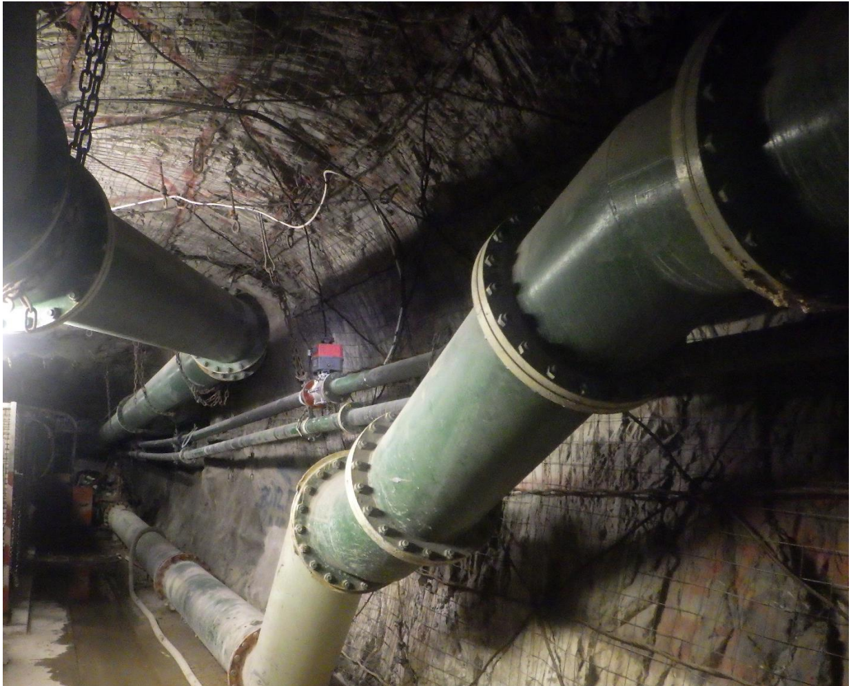
Figure 37: Chilled water distribution columns 3
