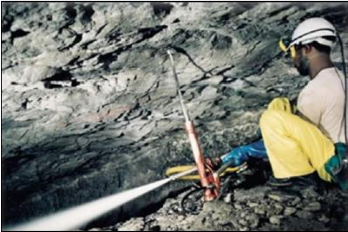
Figure 11: Water cannon in operation [34].
