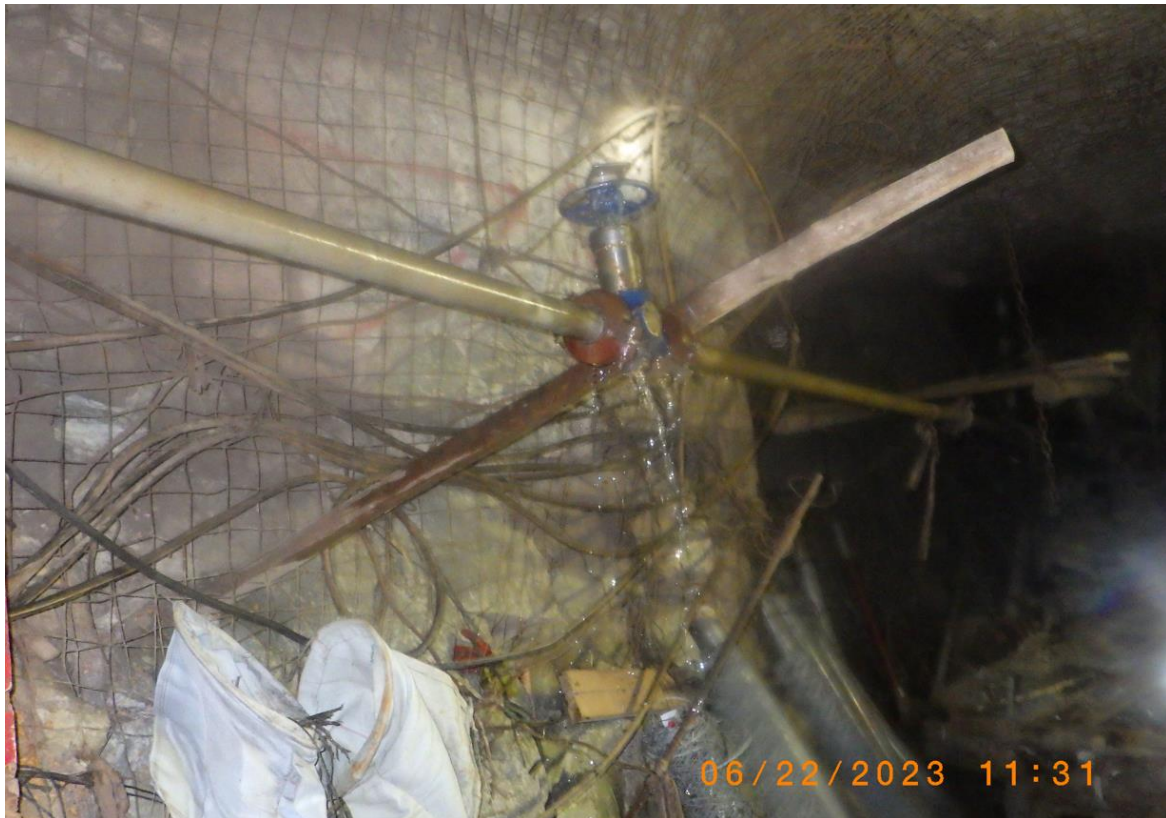
Figure 55: Leaking valve found at the entrance of a working area.
