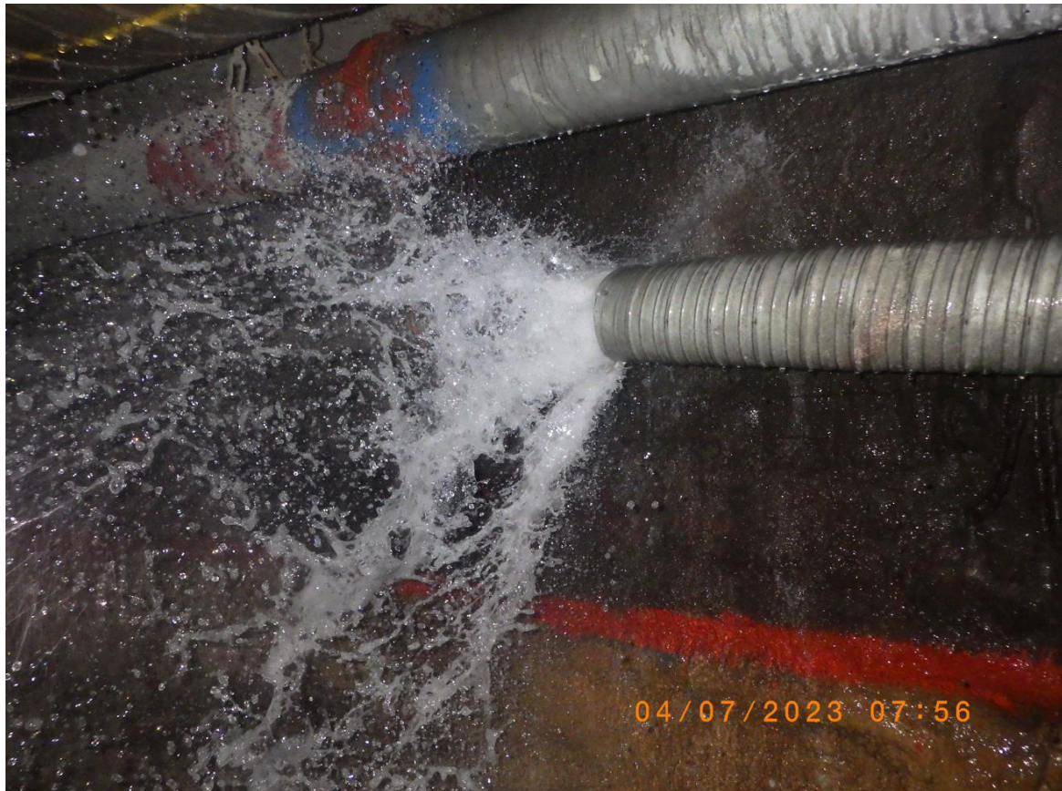
Figure 56: Column burst identified during implementation.
