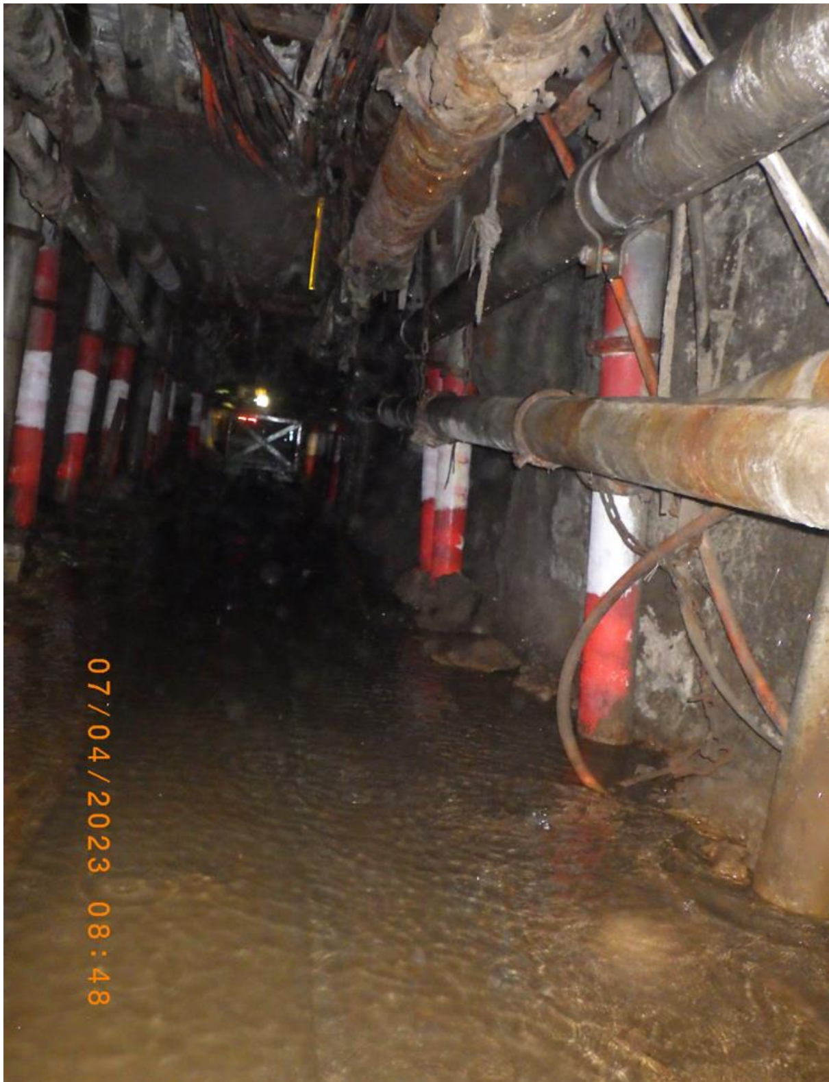
Figure 57: Flooded area as a result of a burst pipe.
