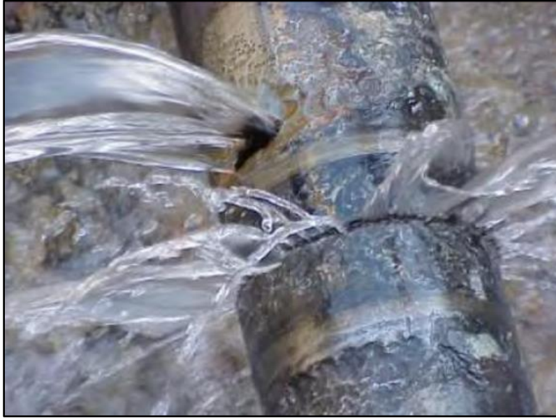
Figure 22: Water leak on steel pipe [28].
