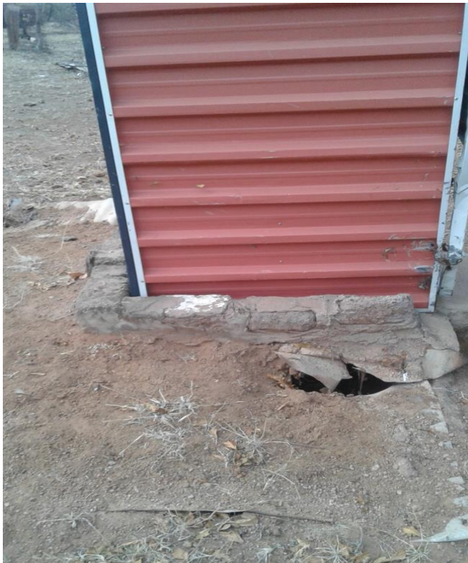
Photo 4: Old pit latrine with no concrete slab
