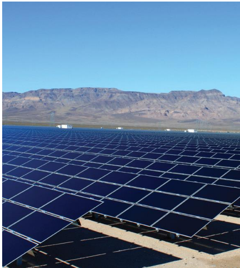
Figure 6.5: Solar photovoltaic (PV) array
