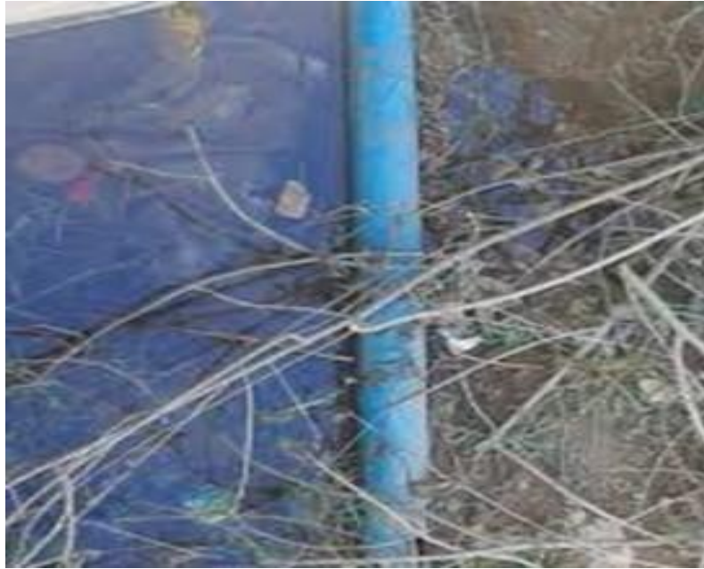
Figure 11: Unattended water pipe leakage.
