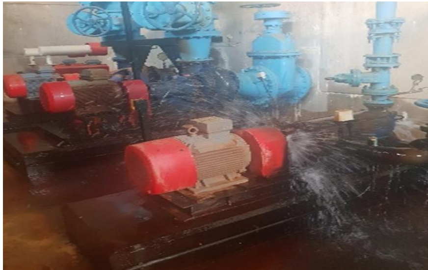
Figure 10: Water leakage from damaged booster pumps.
