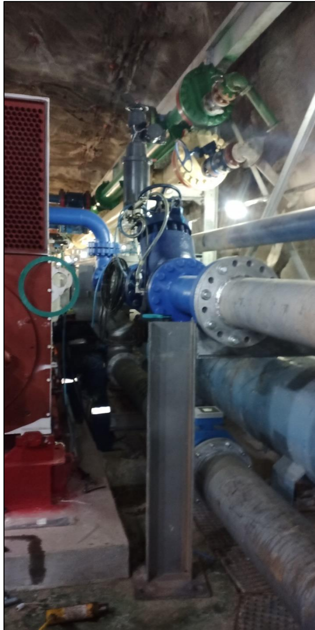
Figure 79: Installed inlet and outlet configuration of PAT
