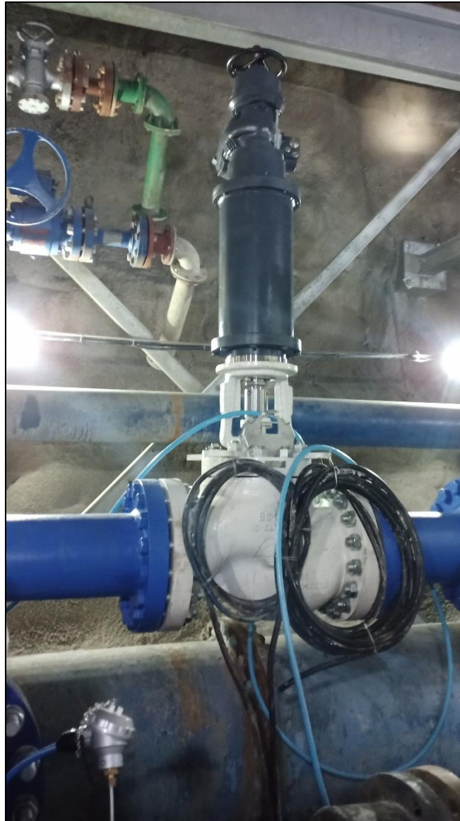
Figure 78: Installed control valve for PAT
