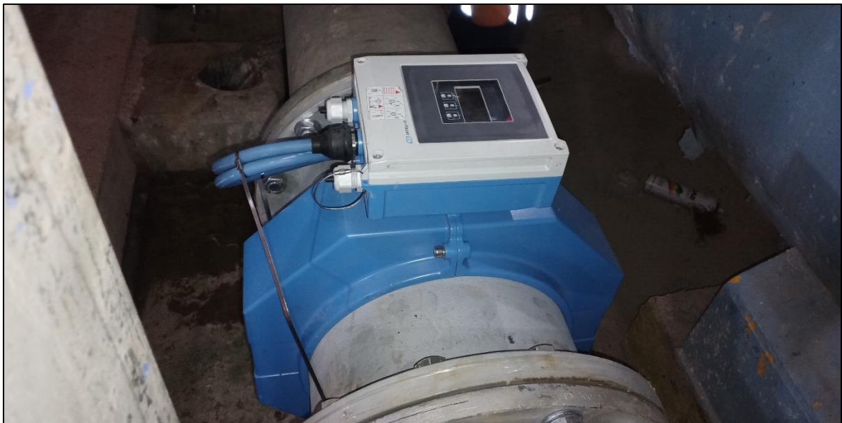
Figure 77: Installed flow meter for PAT
