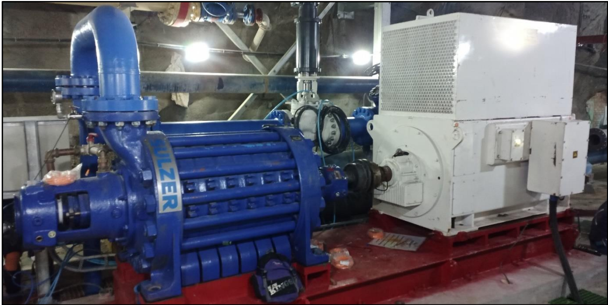
Figure 76: Installed and operational PAT and generator
