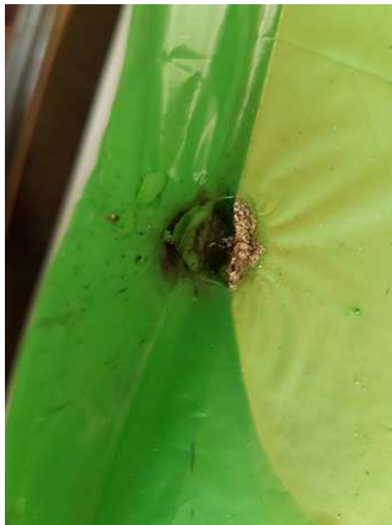
Figure 5-1: Cross-over arcing in a capacitor.
