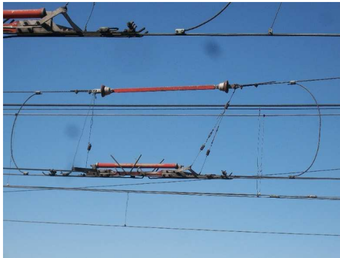
Figure 1-1: An old Mark I 3 000 V DC section insulator.
