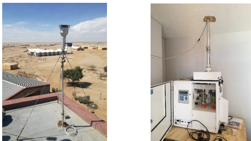
Figure 2-5. The PM 10 inlet on the rooftop of the HBAO connected by a straight stainless steel pipe to the Partisol in the room below.
