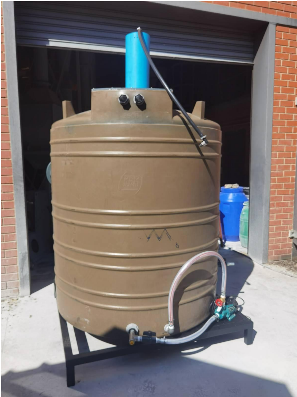
Figure M4: The scrubber
