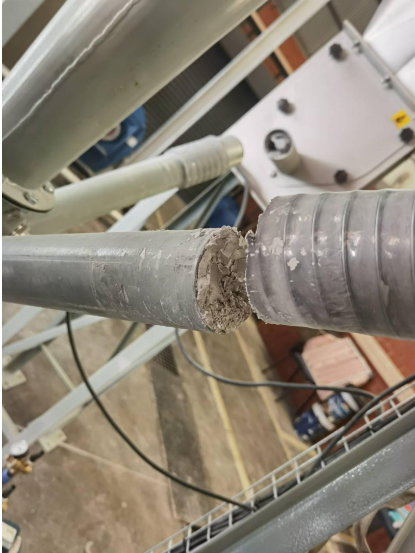
Figure M9: Clogged feed pipe during operation
