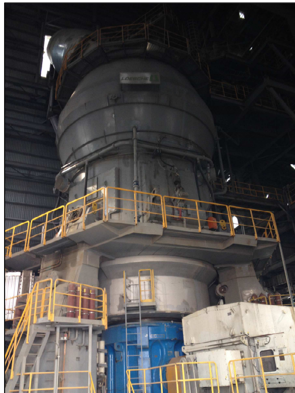
Figure 2-4: Photo of a modern Loesche vertical roller mill XIV
