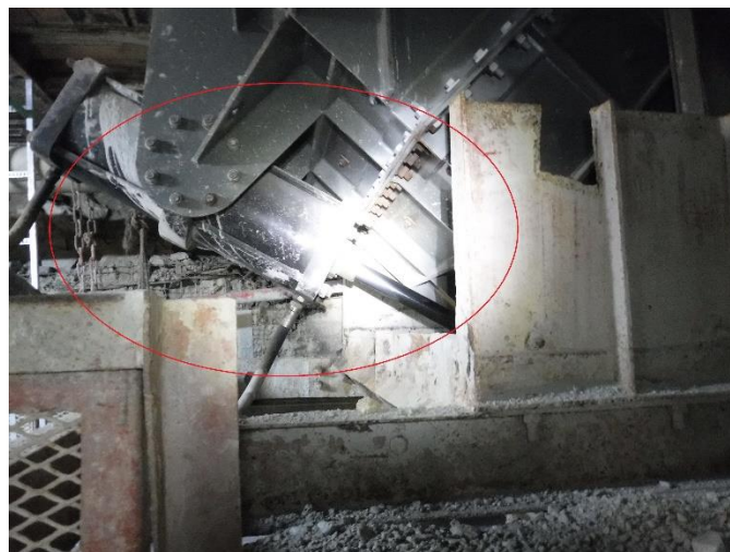
Figure 7: Pneumatic cylinder operating a loading box 1
