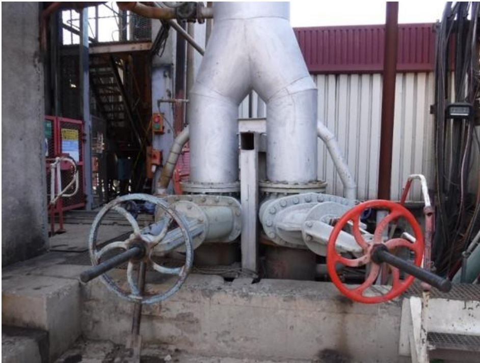
Figure 15: Manual compressed air valves on the surface 4
