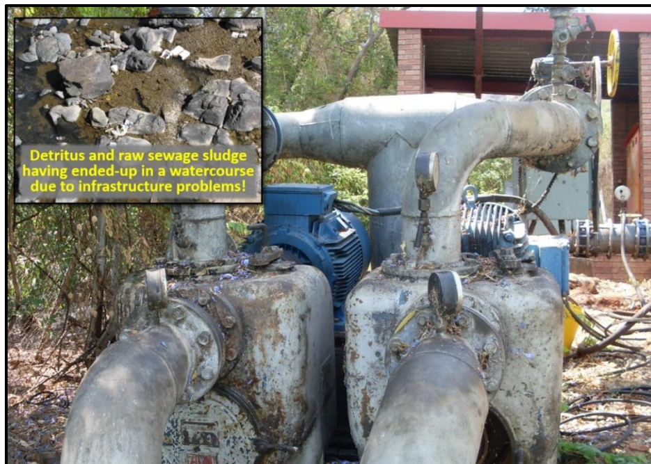
FIGURE 40: Vandalism, ageing infrastructure and insufficient maintenance of sewage infrastructure cause water pollution, which contributes to eutrophic conditions in receiving water resources.
