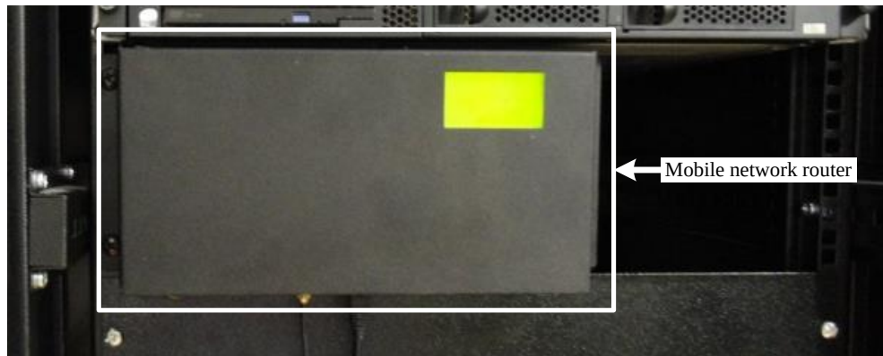
Figure 26: Emulated EMS mobile network router installation
