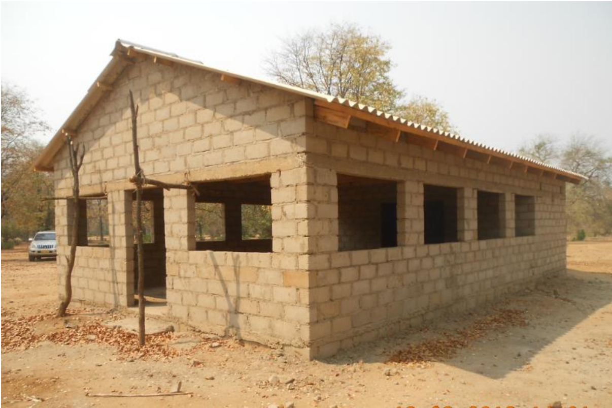
Figure 7-1: ECD Classroom block under construction in the Mahenye village ( Photo courtesy: Owen Gohori )
